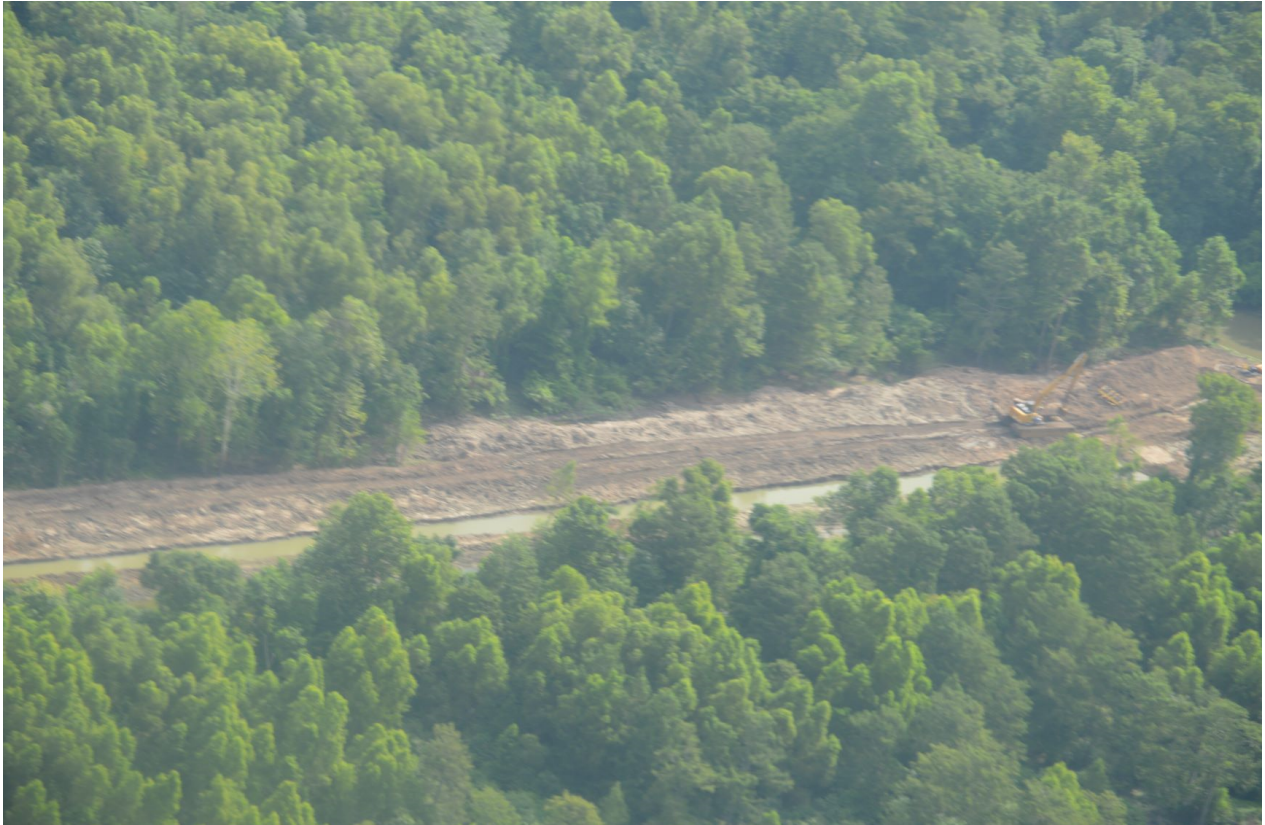
Figure 3. This photo was taken by Dean Wilson during a monitoring flight on July 23, 2018. This photo depicts the pipeline right of way as it crosses the Property. As seen in the photo, there is equipment on the Property and it appears that the trench in which the pipe will be laid is being dug along the pipeline route as it crosses the Property.
